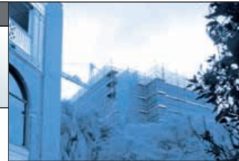
USG Powerscape Health 13mm linings are being used extensively throughout the Mater Hospital renovation and extensions (shown) in Brisbane.
