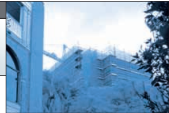
USG Powerscape Health 13mm linings are being used extensively throughout the Mater Hospital renovation and extensions (shown) in Brisbane.
